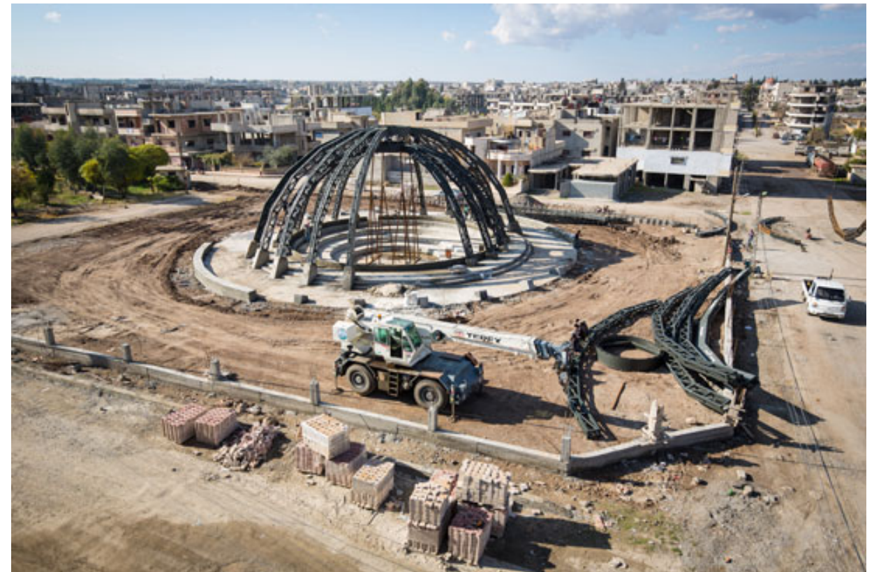
Construction of the new public parliament and surrounding park in the city of Derik, Cezire Canton, in the autonomous region of Rojava in early December, 2015. Photo: Ruben Hamelink/New World Summit.
